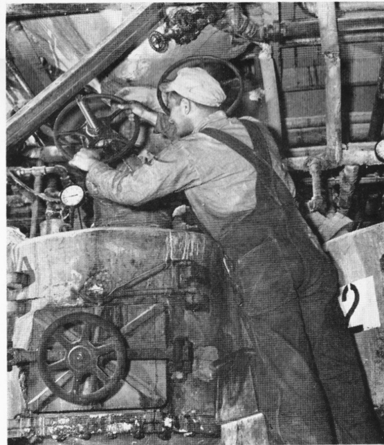
This workman is operating a valve on a salt removing mechanism in a glycerin plant. Thus your household fats become an important chemical for making medicine and ammunition. OWI Photo
